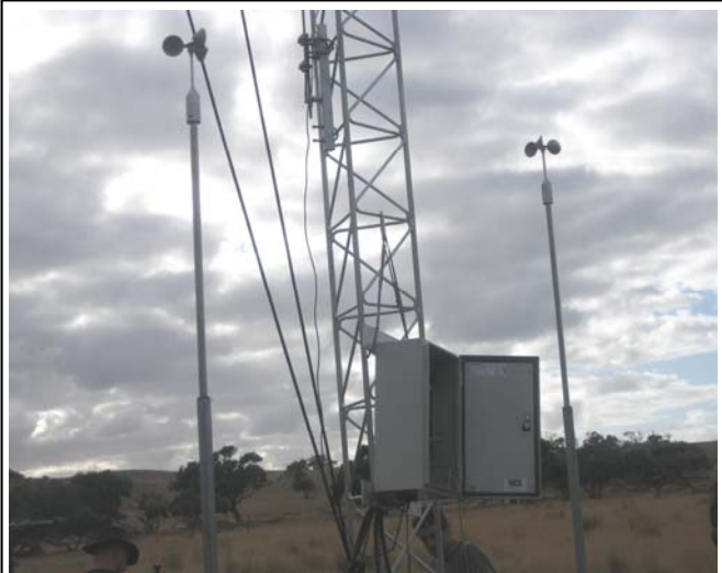
The newly erected meteorological mast at the Bald Hills Wind Farm site
